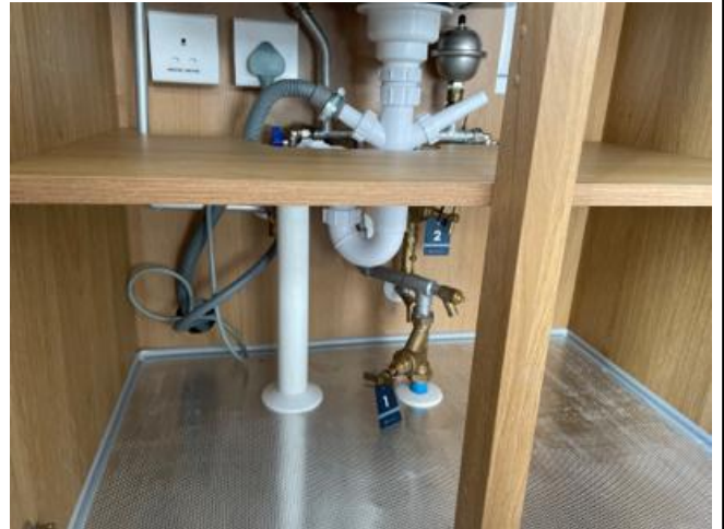
30. Stop cock under kitchen sink.
