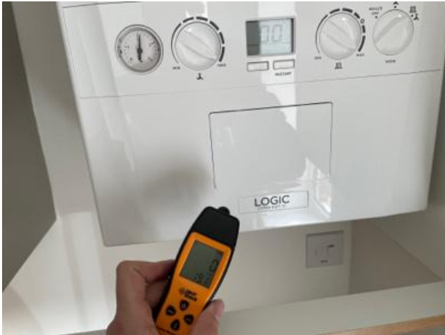
37. CO meter reading.
