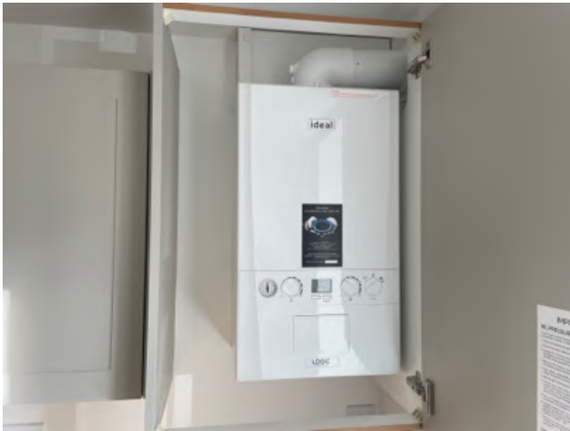
33. Boiler in kitchen.
