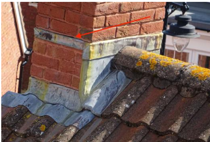
Right chimney mortar cracked
