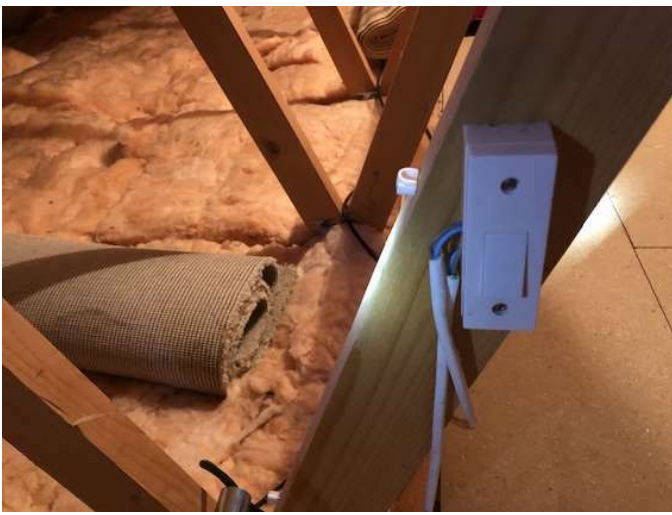
DIY electrics loft
