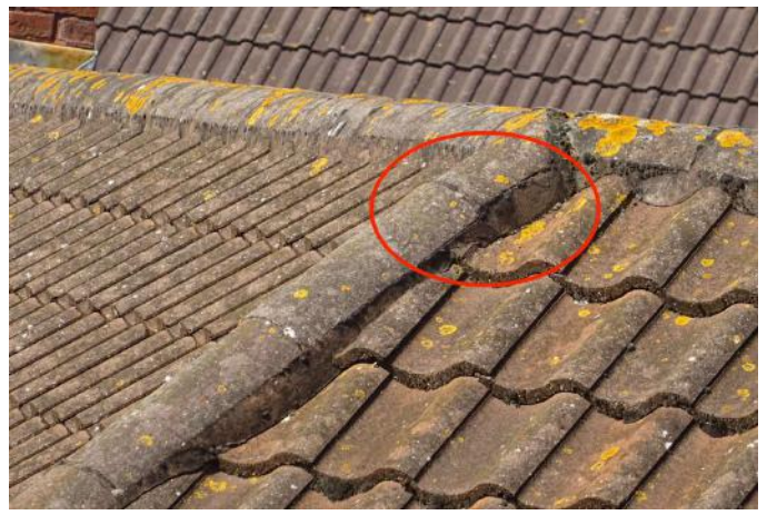
Front hip mortar decay
