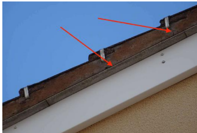
Left verge mortar cracked
