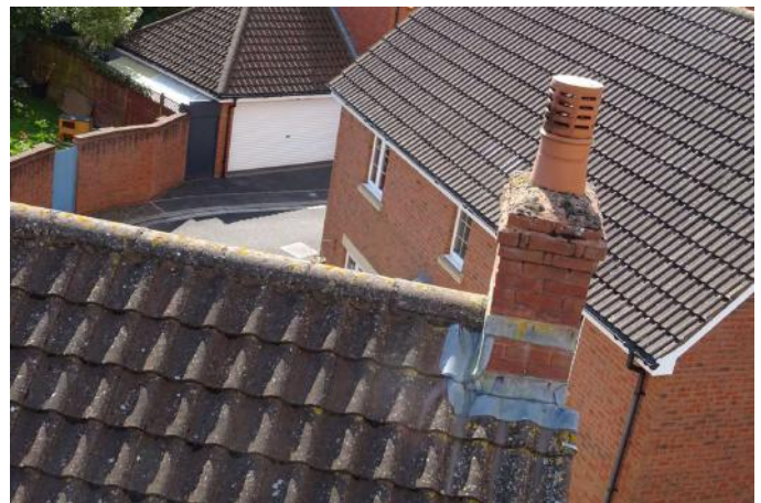
Left chimney moss
