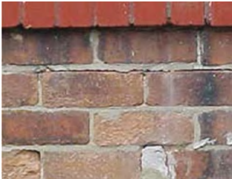
Fig4—Horizontal cracking in mortar joint
