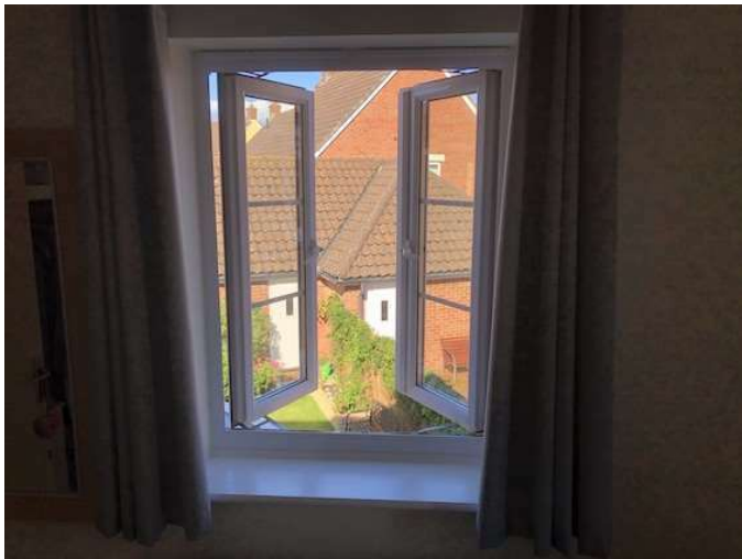
Fire escape window
