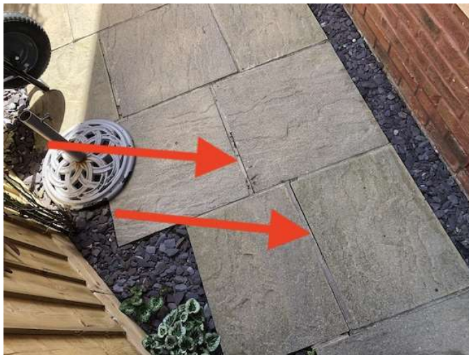
Patio grout failed
