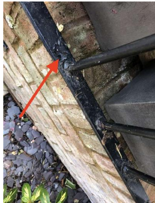
Railings paint failed
