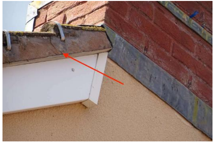
Right verge mortar cracked
