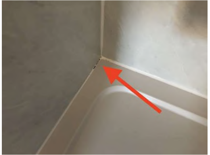
Shower sealant mould
