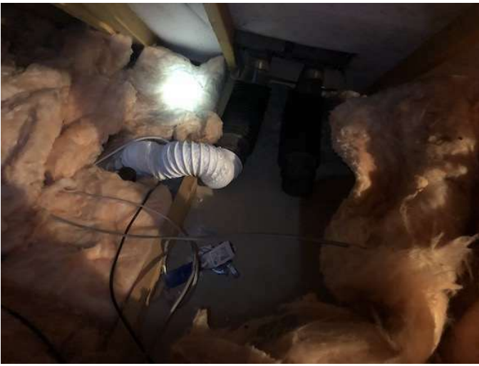
MEV Ducting loft
