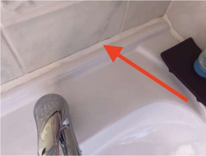
Sink sealant failed
