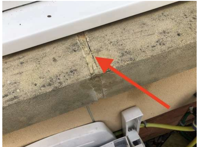
Window cill mortar cracked
