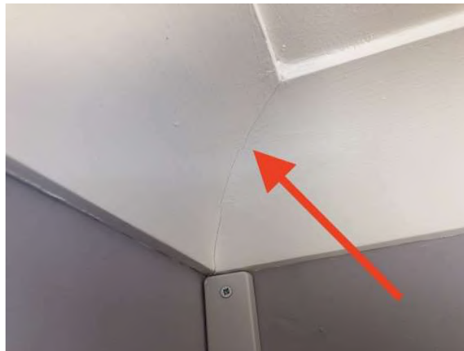
Ceiling thin crack
