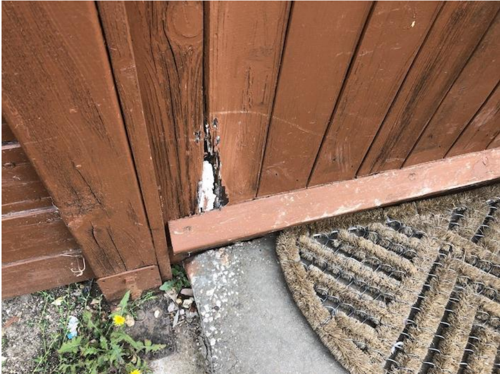
Front door rotten timber
