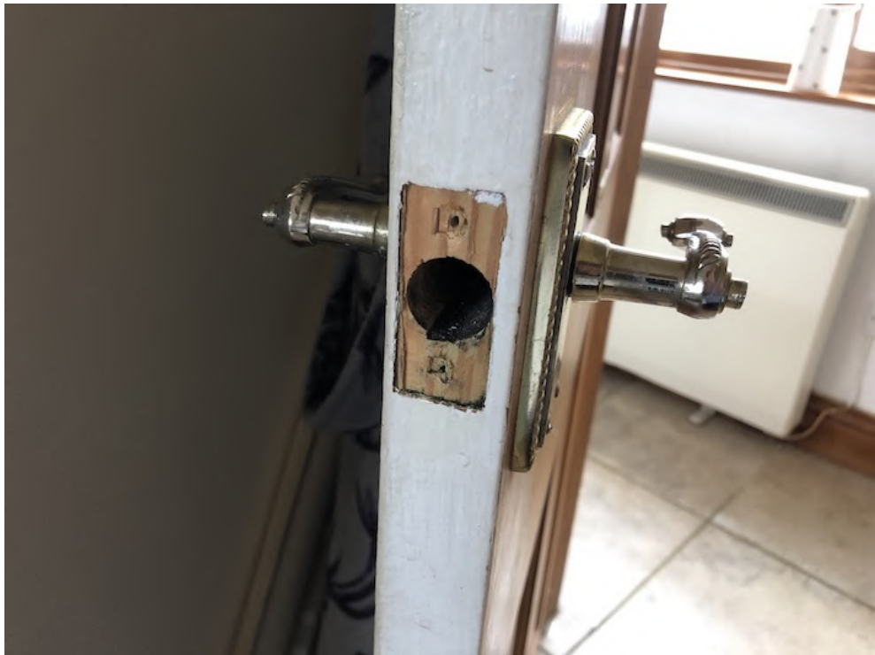
Bathroom missing door lock
