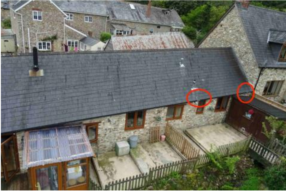
Slipped slates at rear
