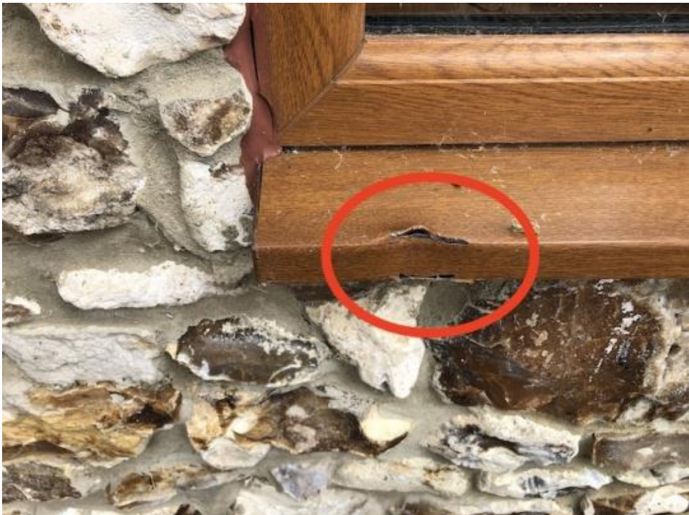
Front left window cill damage
