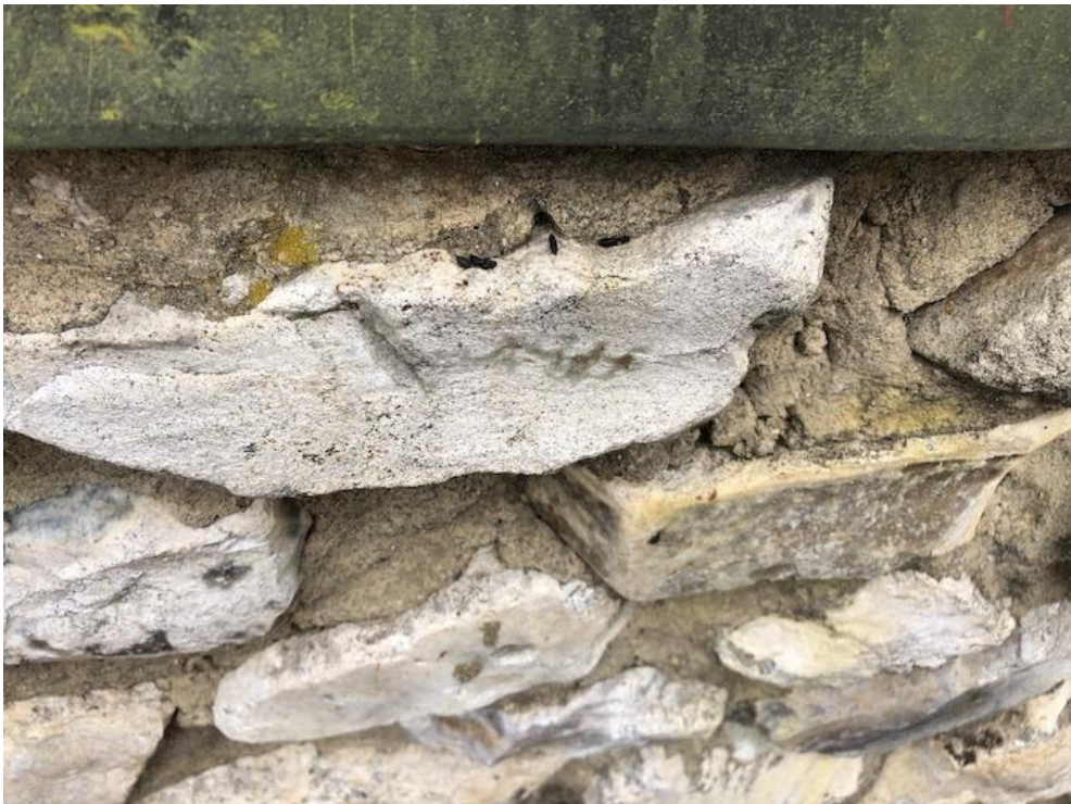
Mortar decay front elevation under right window
