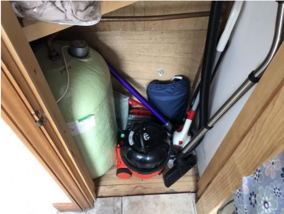
Hot water cylinder
