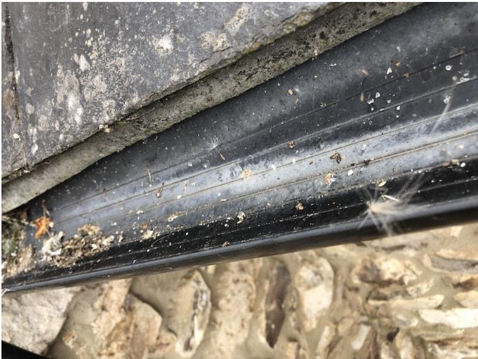
Lack of felt in gutter, this is one of the larger remaining felt areas
