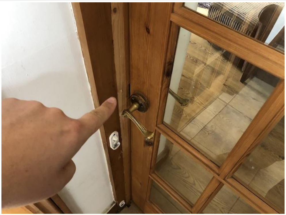
Missing part of door frame
