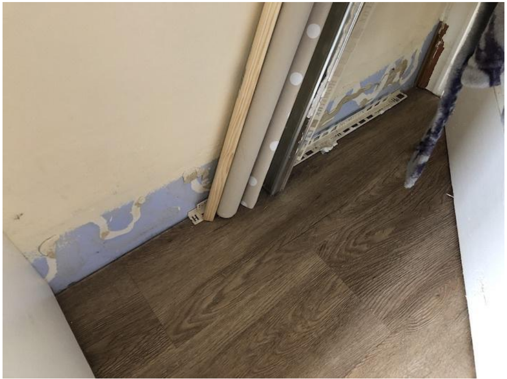
Missing skirting bathroom
