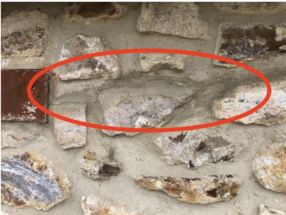
Wall crack rear wall to left bathroom window
