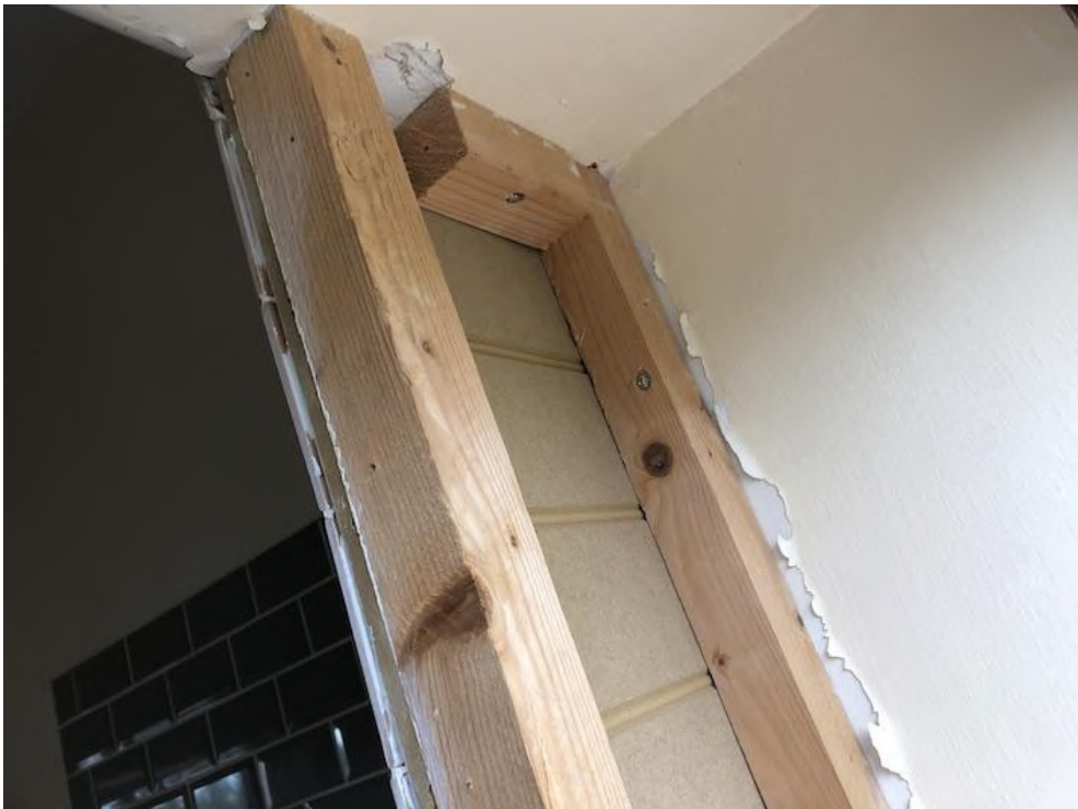
Bathroom shower wall unfinished
