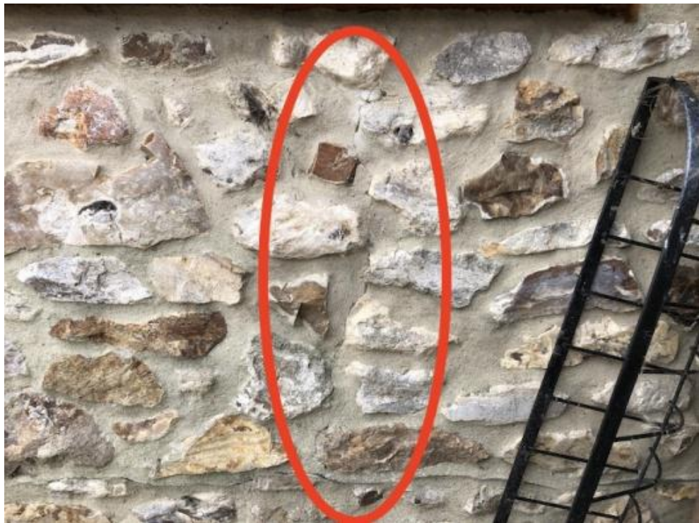
Wall crack rear wall below Bedroom 2 window
