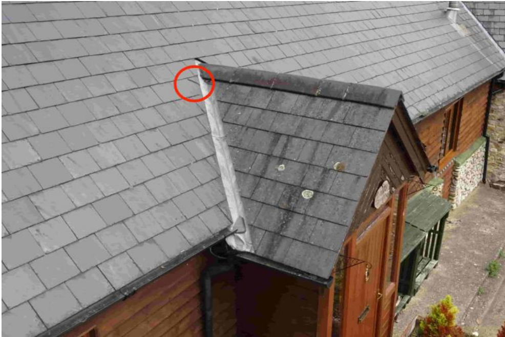
Broken slate to left of porch roof
