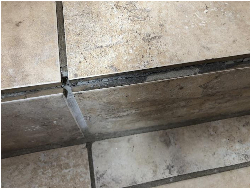
Hallway floor grout
