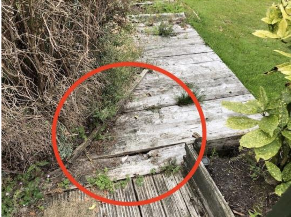
Rear left decking rotten
