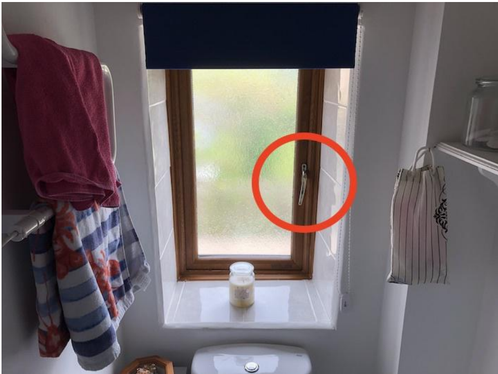
Ensuite window handle loose
