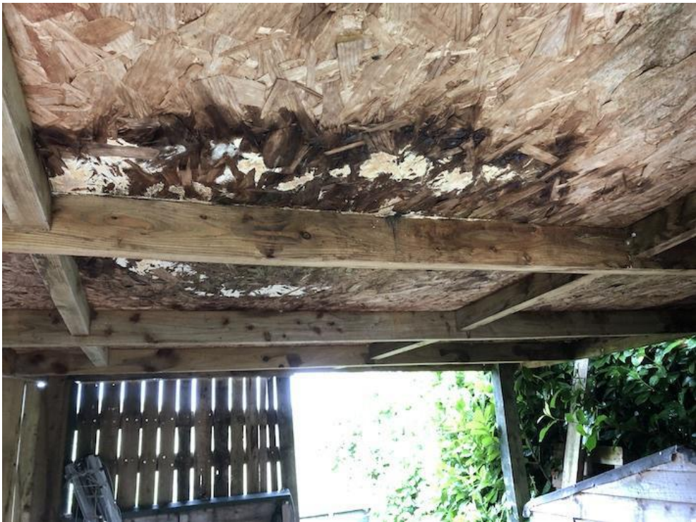
Open shed roof damage
