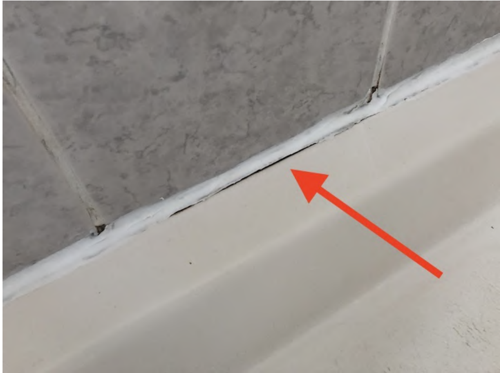
Ensuite shower sealant failed
