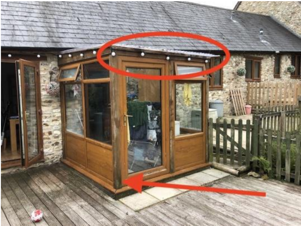
Boot room no gutter and timber defects
