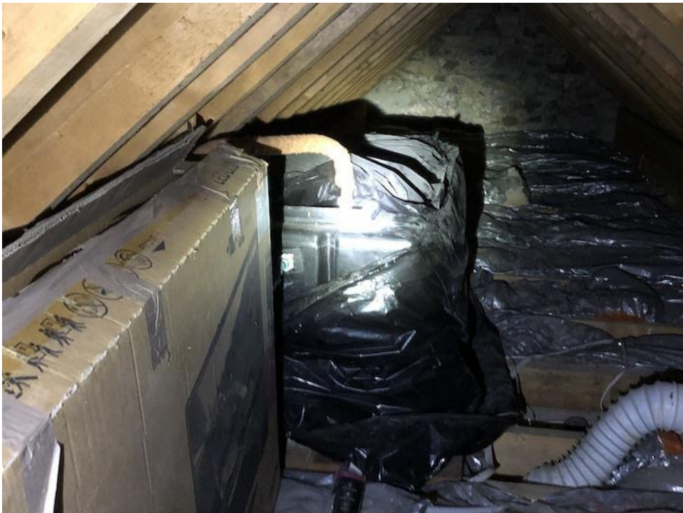
Water tank and loft insulation
